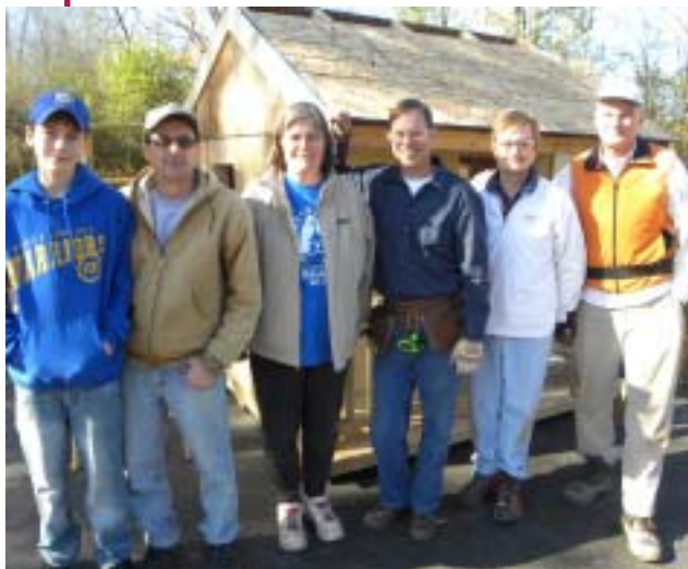
Holy Childhood has a new playhouse, donated and built by the Koinonia Mission Company (KMC) as part of Flower City Habitat For Humanity's Women Build 2011. The playhouse was a practice build before the group attempted a full-size house in Rochester this past year. Our students will make sure it is appreciated for all the hard work that went into it!
